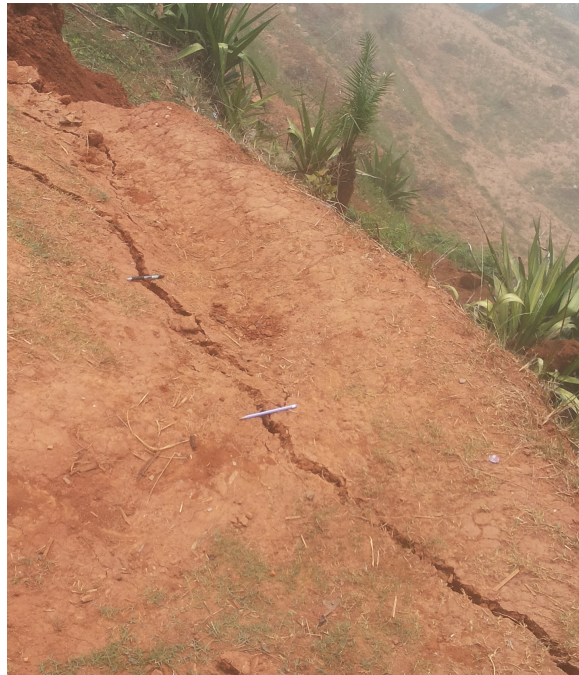
Figure 5: One of the cracks on the western face of Bisteutar village hill.
