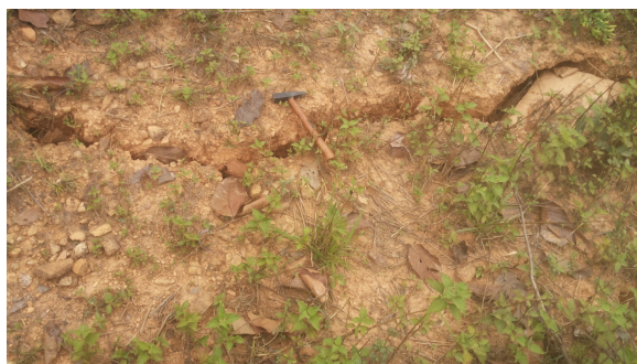
Figure 7: One section of the crack that runs along the length of the Jhyadi village hill.
